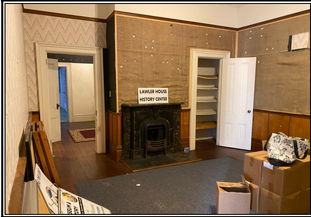
Interior of ground floor space, water damage in the closet is evident with the warped boards.
