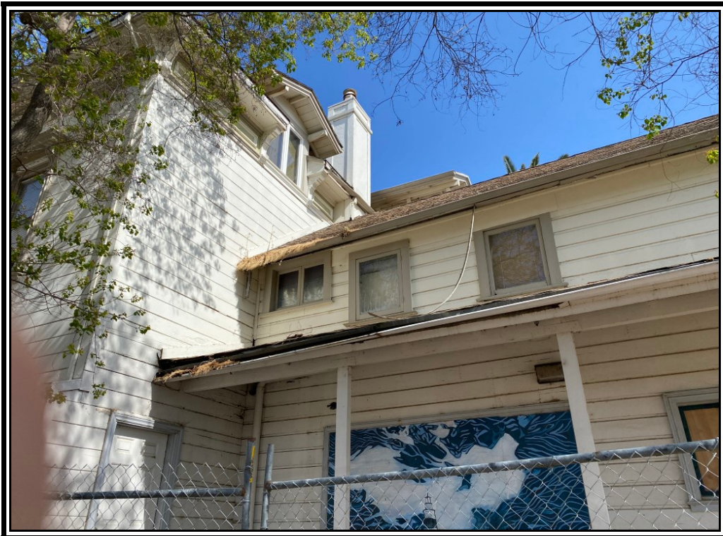
South side of the building which shows extensive roof and gutter damage. Note that both gutters in image are failing and show signs of vegetation growth that typically is associated with a build up of organic material over multiple years.
