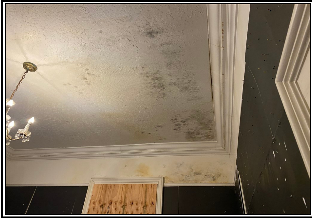
Extensive mold was found throughout the property as is evident on the roof and walls in this image.
