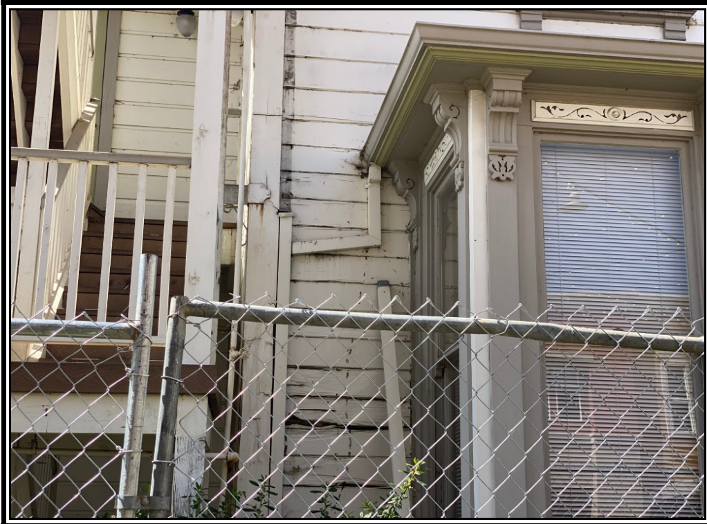
On the northern side of the building there are multiple gutters and down spouts that are no longer connected, resulting in water damage to the siding as is seen in this image. This lack of down spouts and gutters has also allowed water intrusion into the core of the building.
