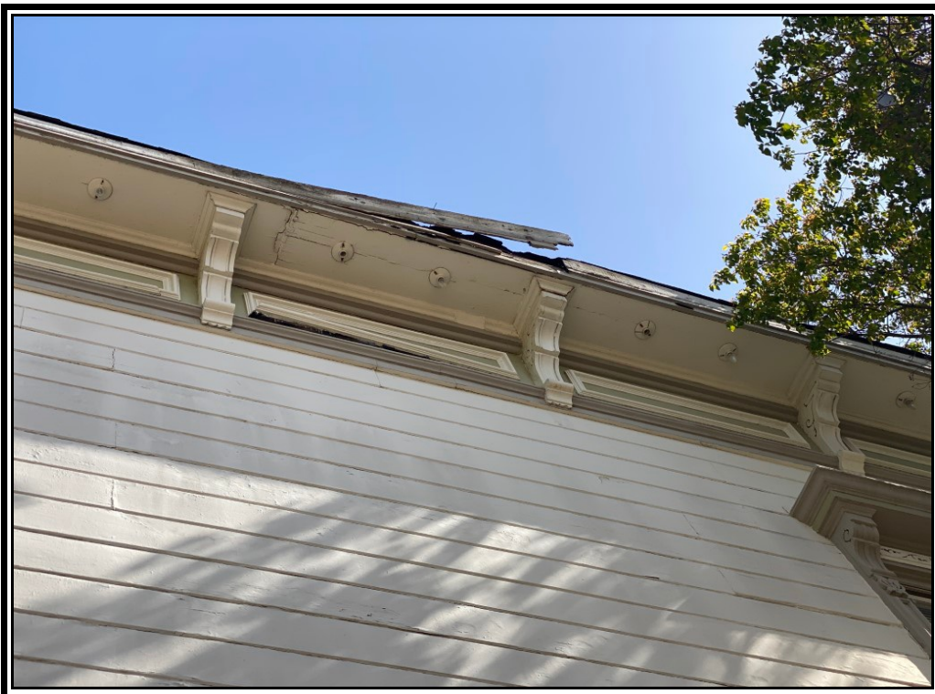
Additional exterior damage to roof trim. Extensive dry rot is visible all around the building.
