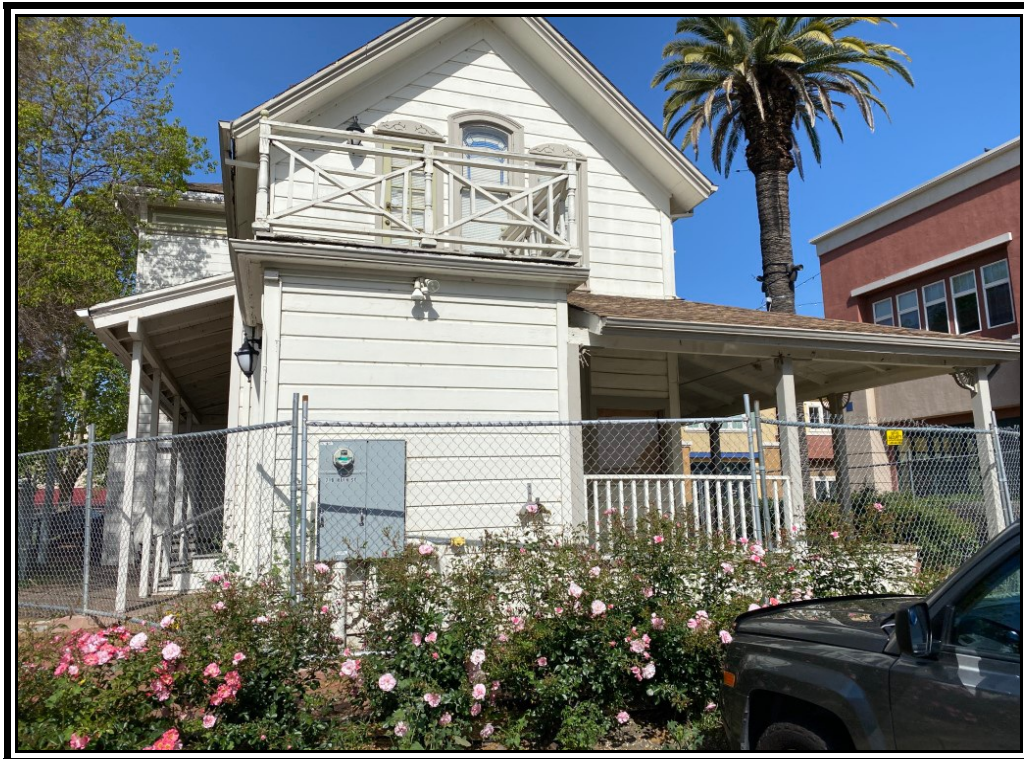
Rear of the building with 2 nd floor deck that was reportedly unsafe to access.
