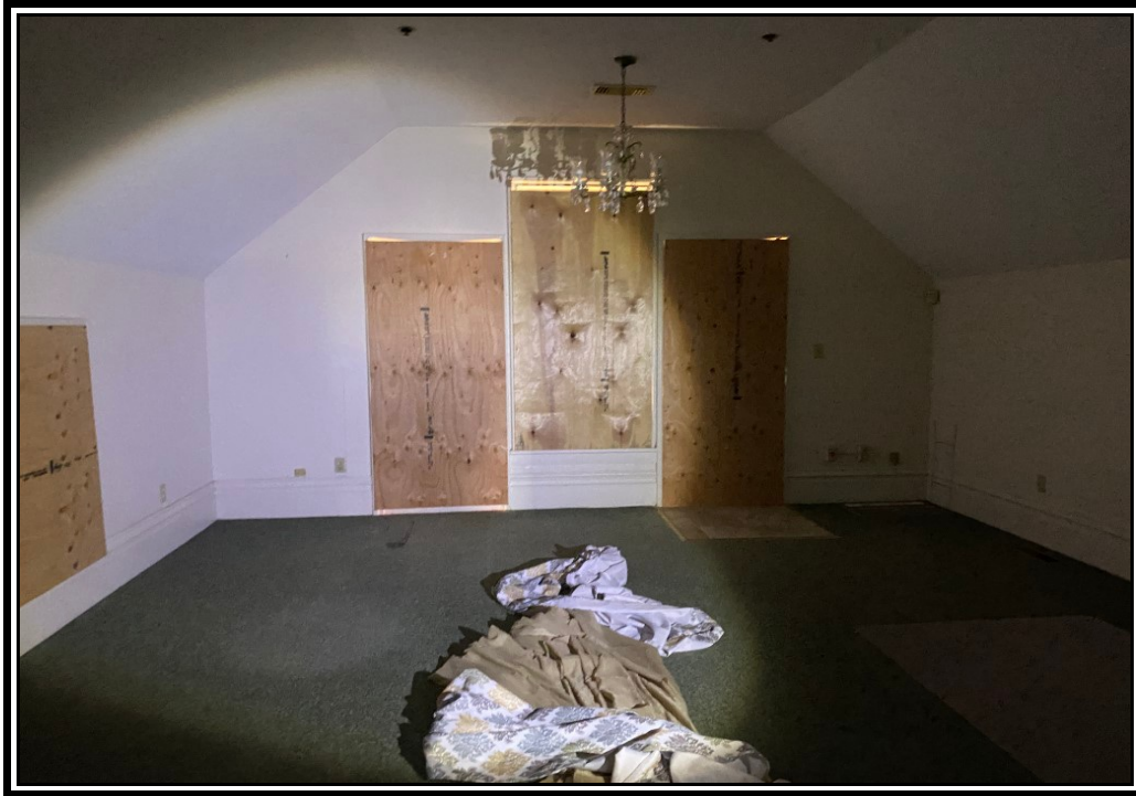
2 nd floor space with non-market standard ceilings that limit the function use of the space.
