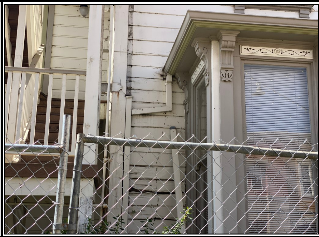
On the northern side of the building there are multiple gutters and down spouts that are no longer connected, resulting in water damage to the siding as is seen in this image. This lack of down spouts and gutters has also allowed water intrusion into the core of the building.
