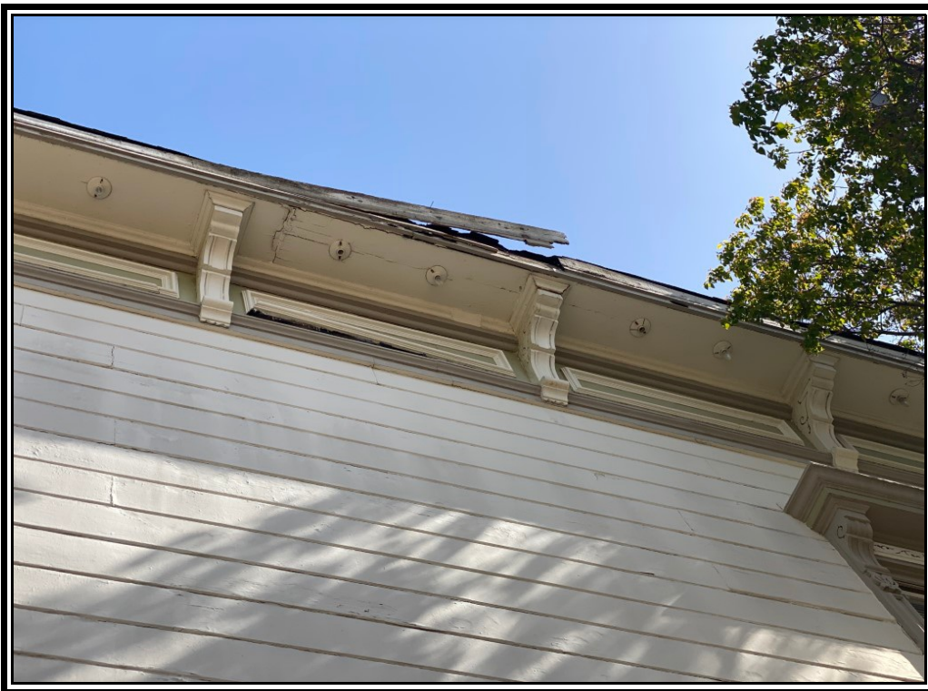
Additional exterior damage to roof trim. Extensive dry rot is visible all around the building.
