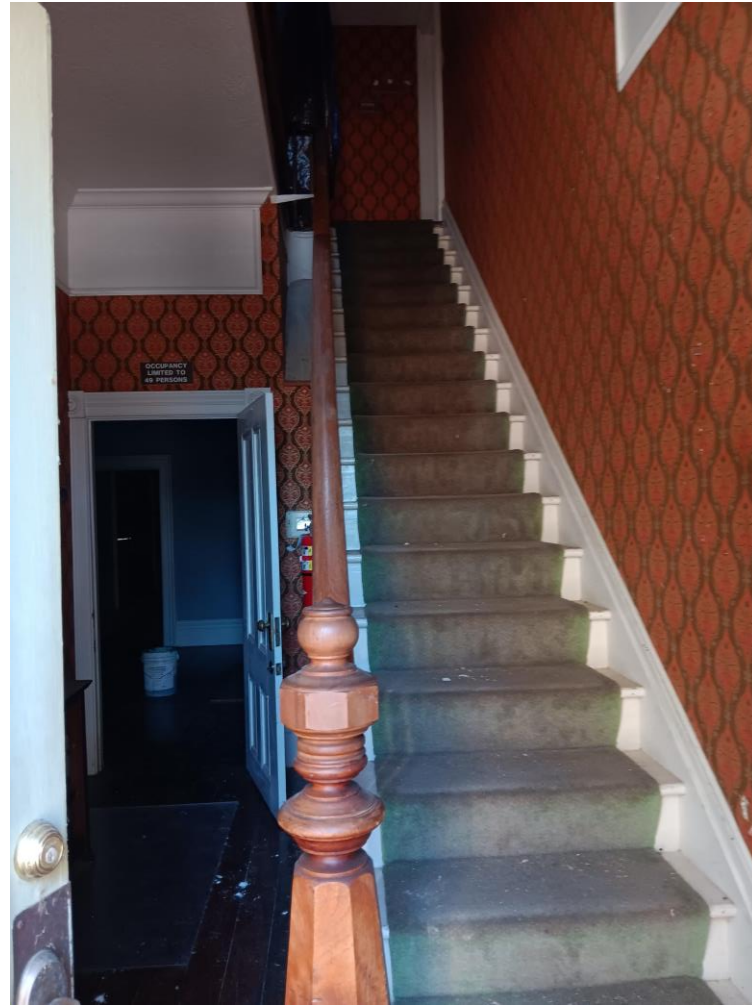
Water damage on stairs
