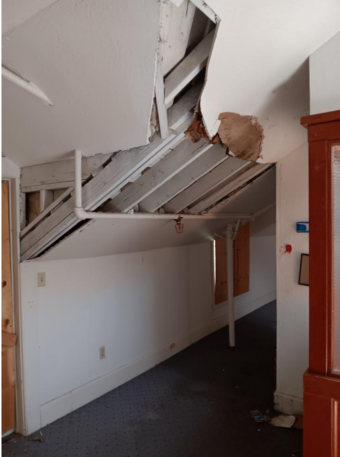
Water Damage on ceiling
