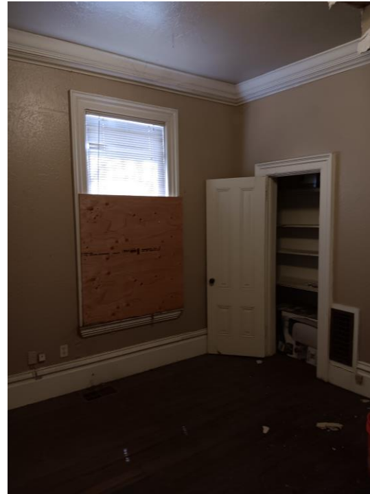
Office 2 (at top of stairs, middle) has water leaks and ceiling damage
