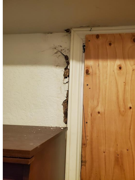
Hallway: Water damage
