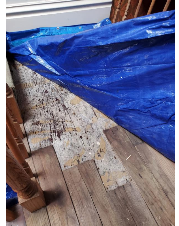
3 rd Story Landing: Water damage & mold
