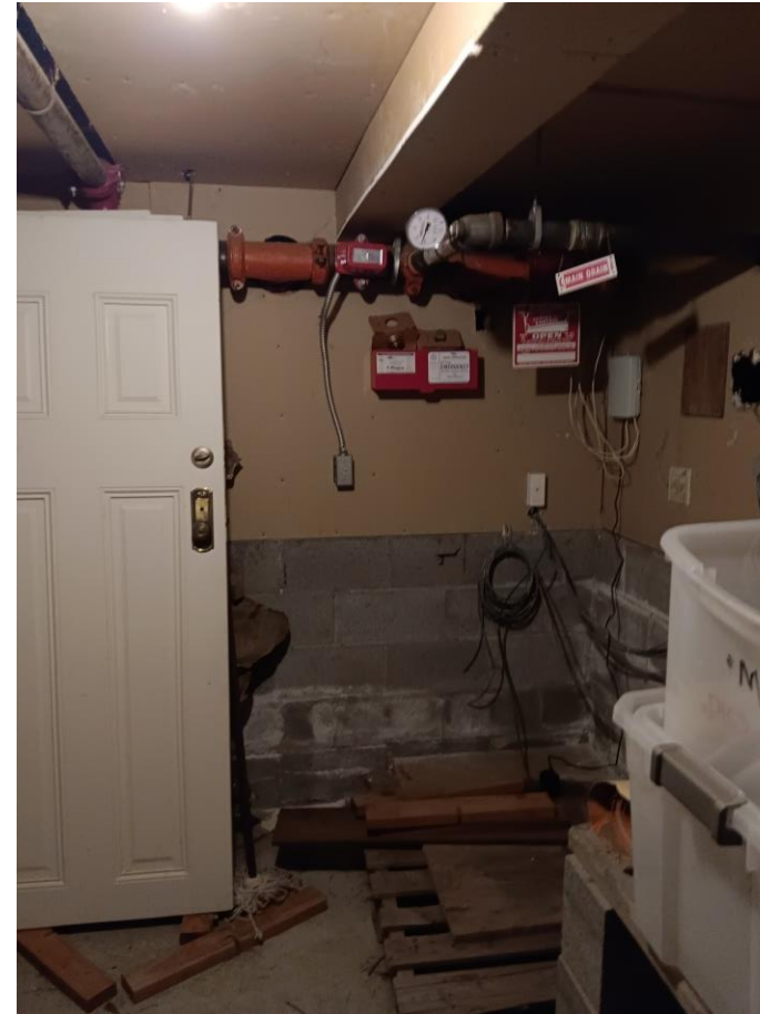
Fire Protection System
