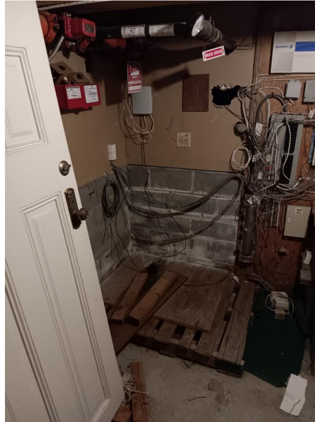
Communication lines & Fire Protection
