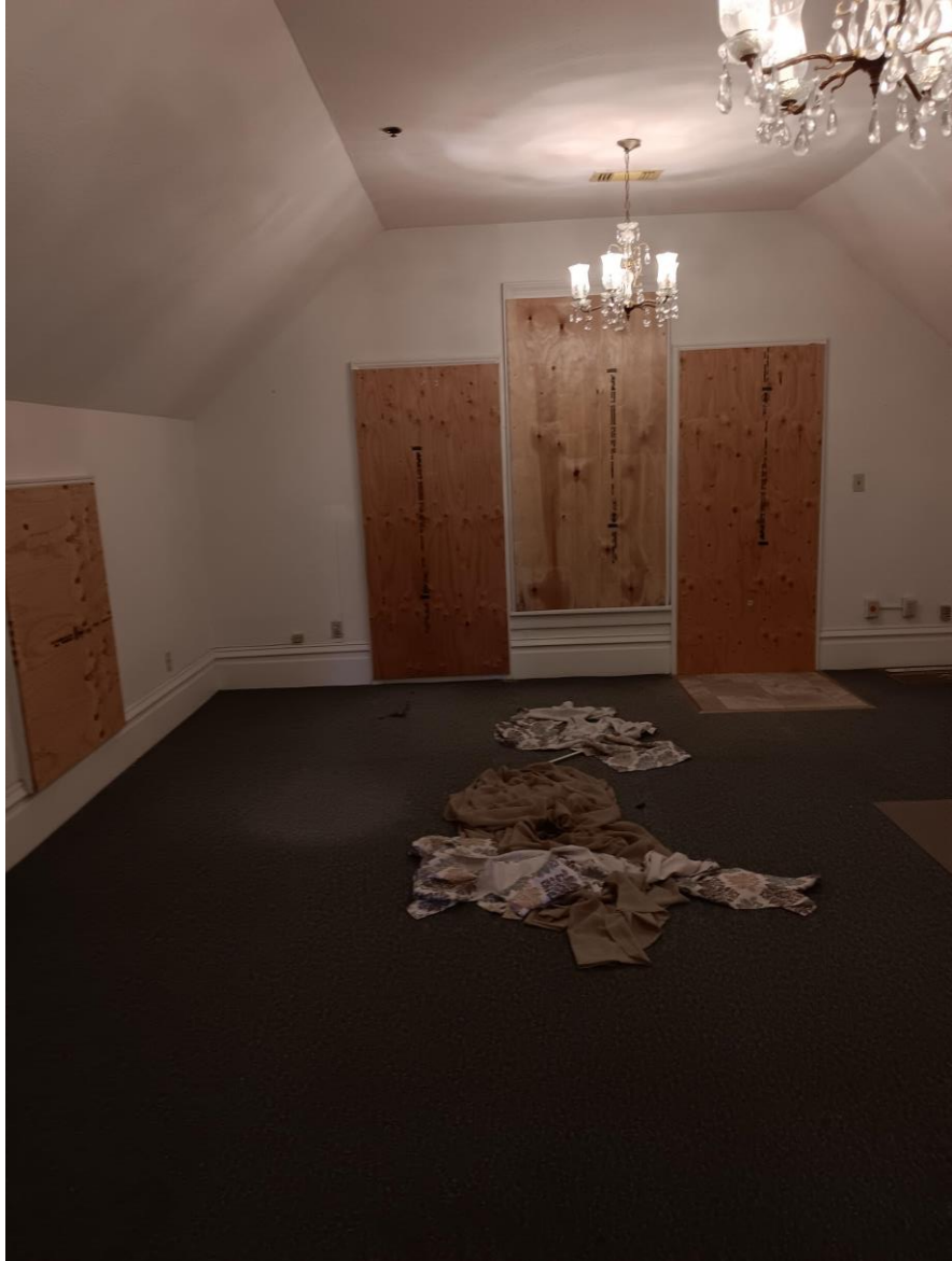
Water leaks and damaged floors
