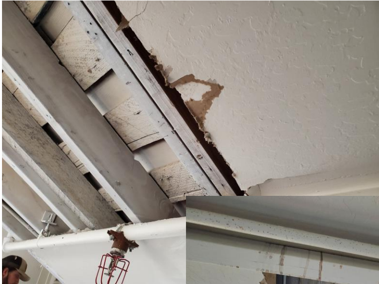
Attic Space water damage under roof
